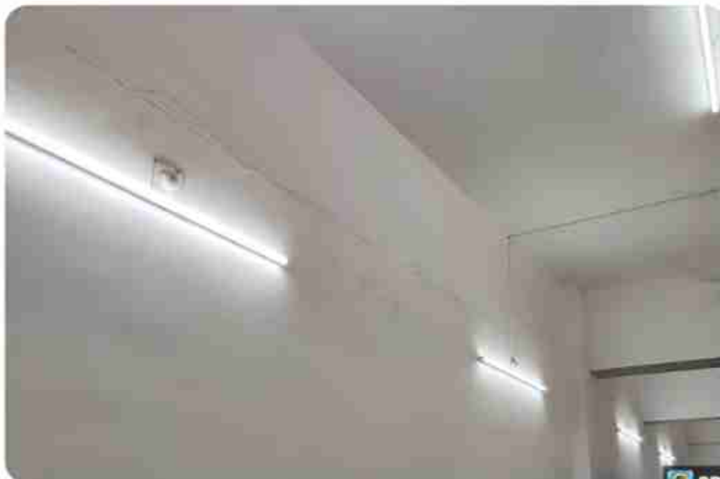
LED LIGHTING IN LECTURE ROOMS AT SAKCHI CAMPUS
