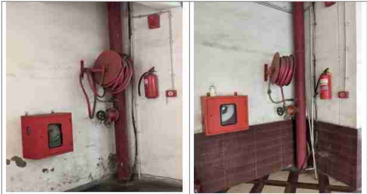
Fire Hydrant with Jockey Pumps
